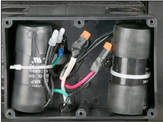
Figure 69. Motor junction box.
